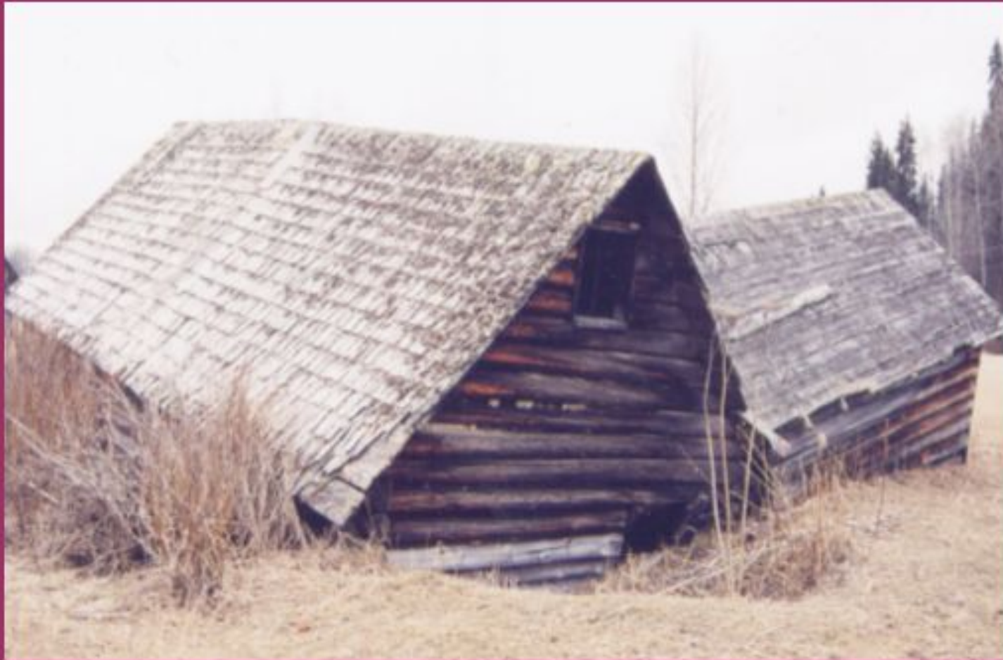
The first Pickering house built circa 1910, slowly disappearing into the ground
